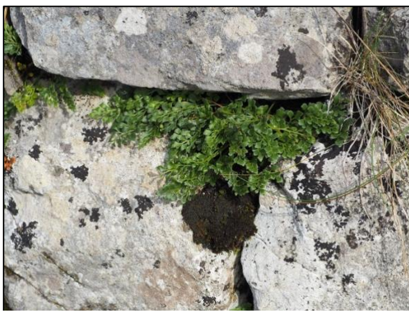
Photograph 5 – Wall rue (a type of fern) growing in stone wall
